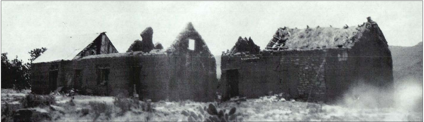
Figure 12: The remains of the main house, as well as those of a house next to it, after it was damaged by a fire.
