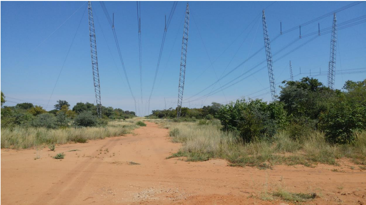
Figure 24: Existing power lines along the proposed routes.
