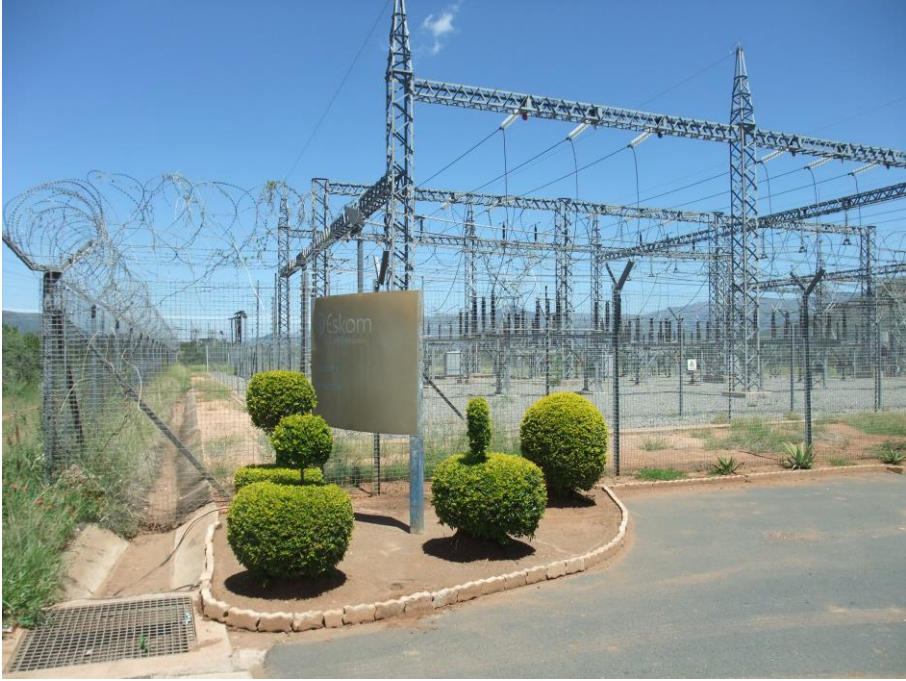
Figure 4: The Mampuru substation.
