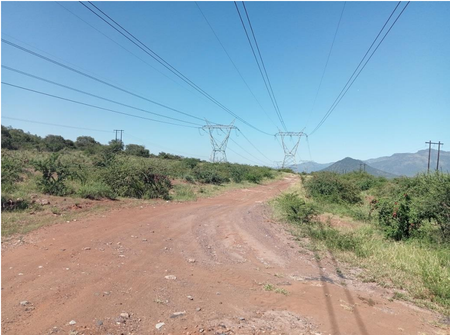
Figure 6: View of existing powerline between points E and G of the deviation.
