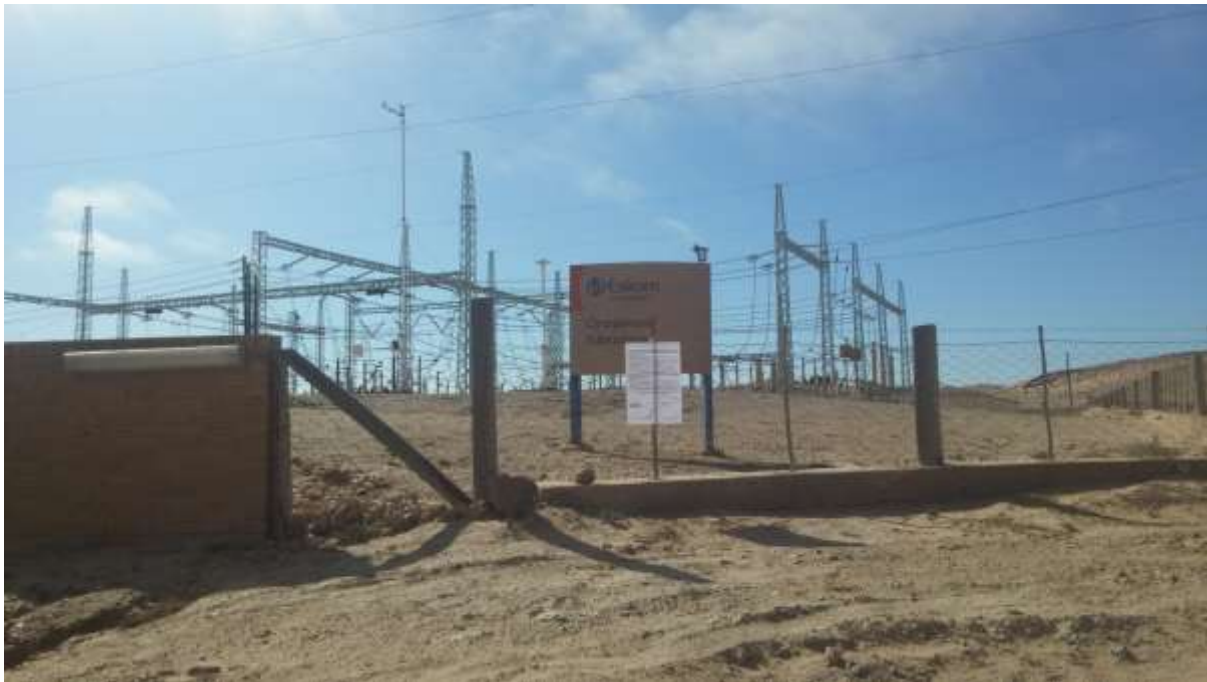
Figure 8: Site notice at the Oranjemond substation.
