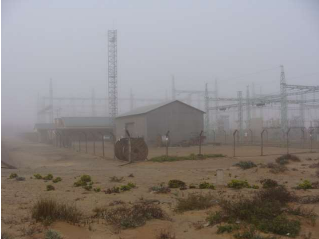
Figure 19: The existing substation in the surveyed area.
