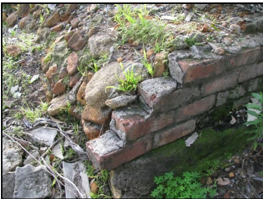
Figure A1.3: Modern brick and stone ruin from west side of site.
