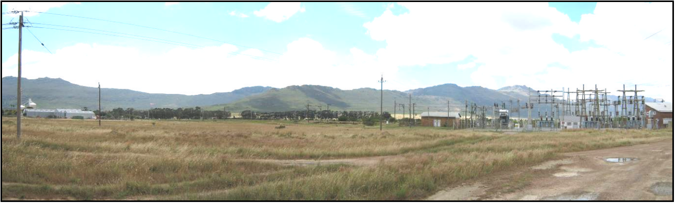
Figure 66: View eastwards of the Gouda substation.
