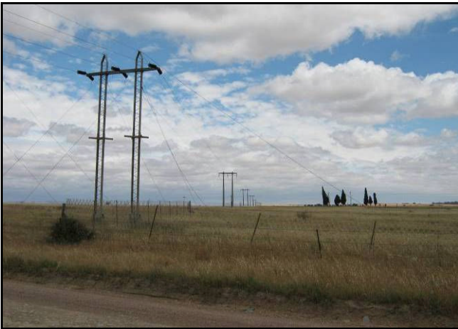
Figure 67: Power lines west of the Gouda substation.
