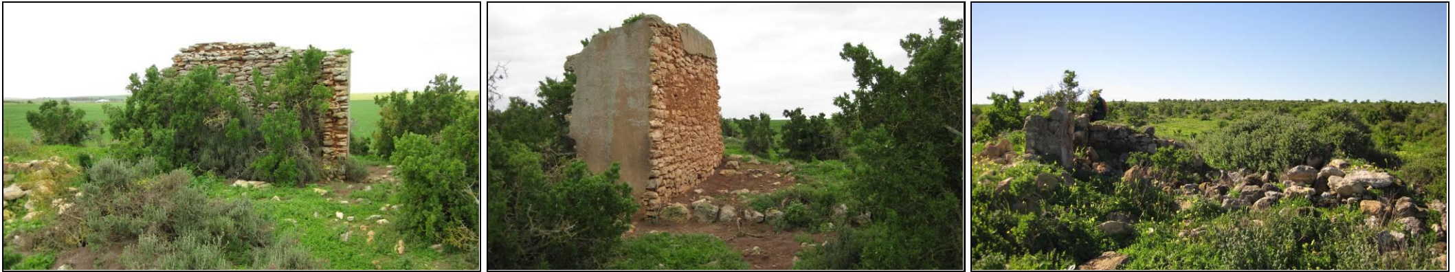
Plate 21 & 22: Historic structures use the abundant limestone chunks as building material with mud used as a binder. More recently, a cement skim was applied to the outer surfaces to prevent rain damage. This building (007) is not directly threatened by the activities. It is of moderate interest only. Plate 23: A small cottage (051) is built in much the same manner as (007). Both 007 and 051 may have been old farmhouses.
