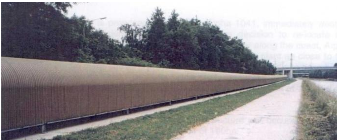
IBR covered conveyor belt system
