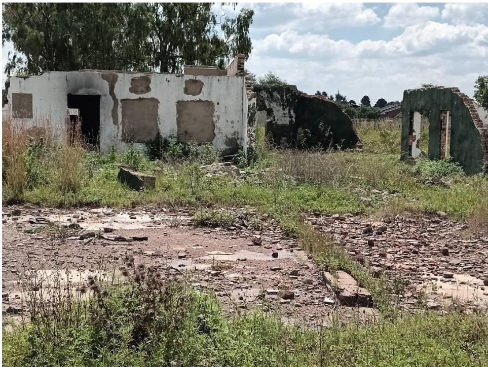
Figure 79: Another view of the ruined structures
