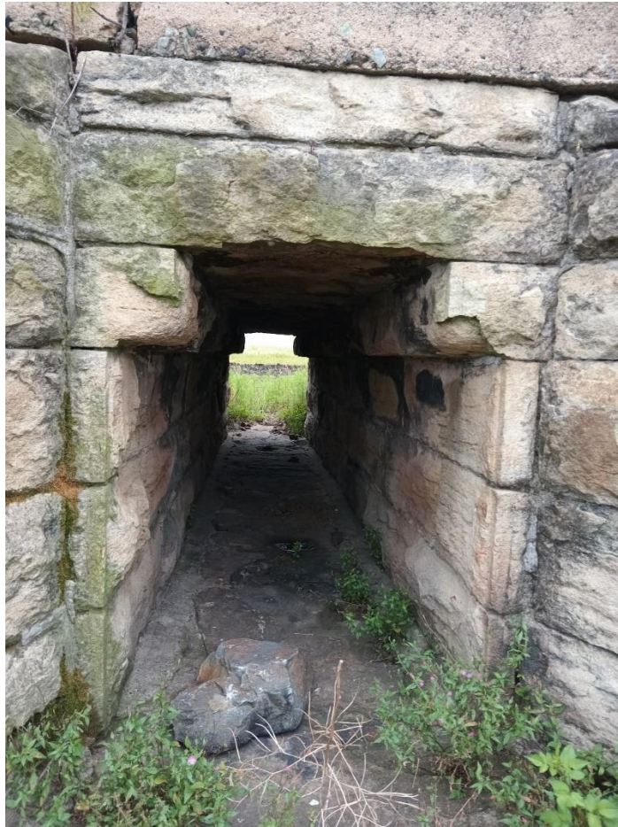
Figure 28: View of the stone culvert under the railway line at CCUS-03. This seems to be an example of a flat lintel or box culvert.
