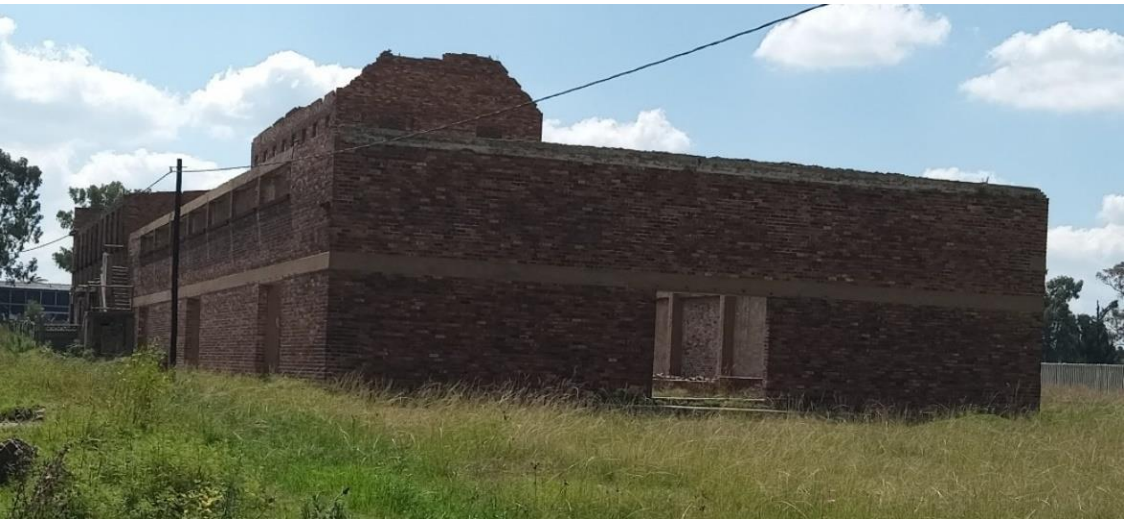
Figure 83: View of another of the dilapidated historical mill buildings
