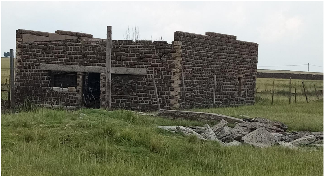
Figure 52: The building built with dolerite stone and sandstone details at the corners and windows, note the demolished material in the foreground
