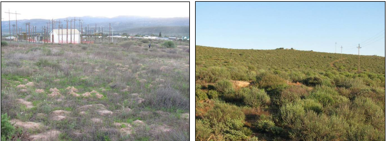
TL: Existing Clanwilliam sub-station. TR: Existing powerline on the north side of Ramskop at Clanwilliam
