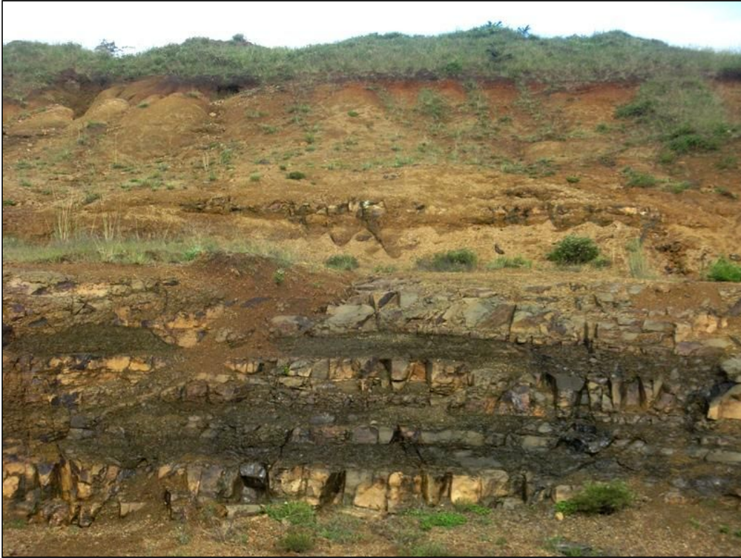
Figure 10. Large borrow pit 600 m west of the R63 near Bisho (Loc. 042) showing thick (> 10 m) zone of khaki-hued saprolite - i.e. in situ weathered bedrocks (Balfour Formation sediments locally intruded by dolerite) - overlying fresher-looking, grey-green, tabular-bedded Balfour beds.
