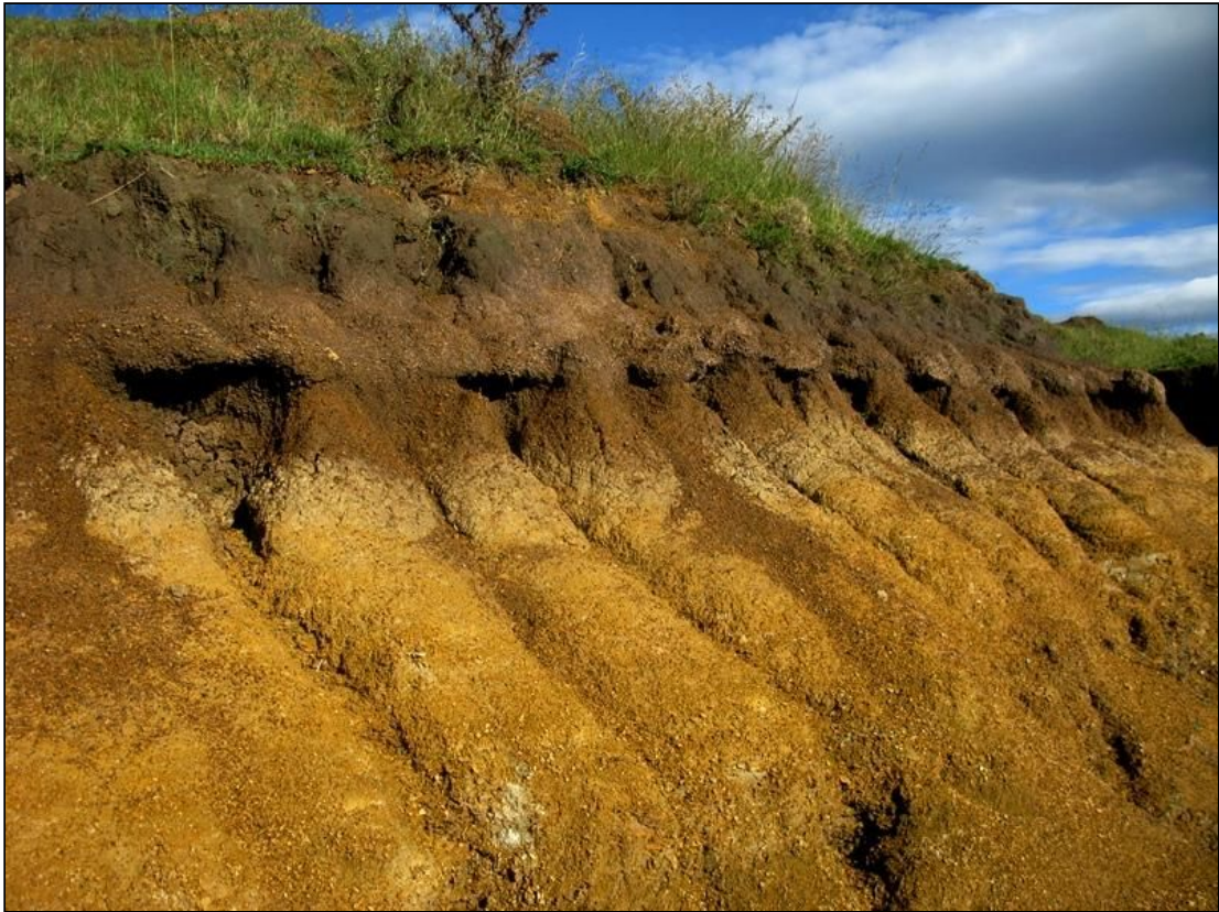
Figure 28: Deeply-weathered, khaki to ochreous Balfour Formation saprolite overlain successively by a thin pallid zone, rusty-brown ferricrete hard pan and dark brown soils, borrow pit west of the R63 near Bisho (Loc. 042).
