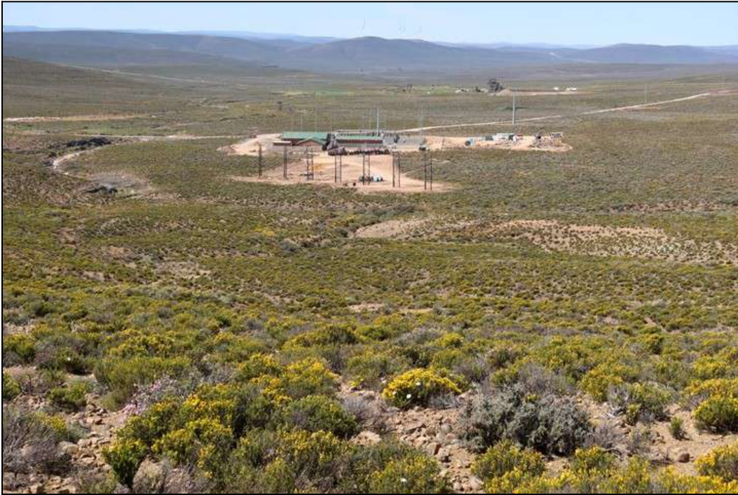
Figure 6: View from the SW towards the new Eskom electrical substation on Bon Espirance 73 with an existing powerline heading eastwards towards the Komsberg MTS adjacent to an upgraded access road.
