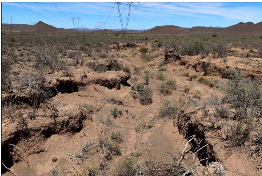
Figure 47: Donga-eroded, thick sandy to gravelly alluvium underlying vlaktes in the main grid connection corridor west of Blouberg, Farm Burgers Fontein 92.
