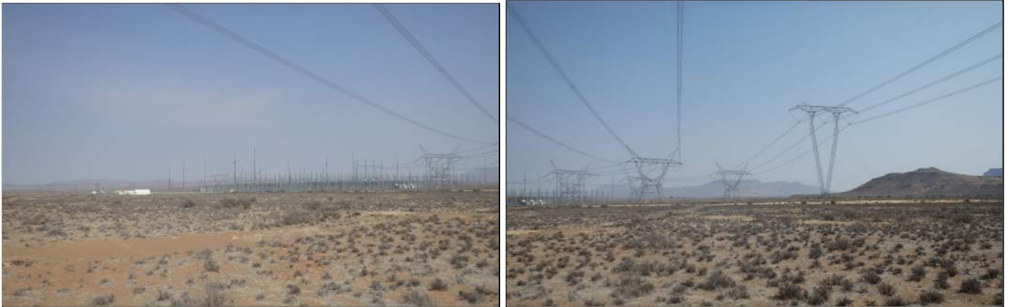
Figure 4.1: Existing grid infrastructure at the southern extent of the proposed grid connections
