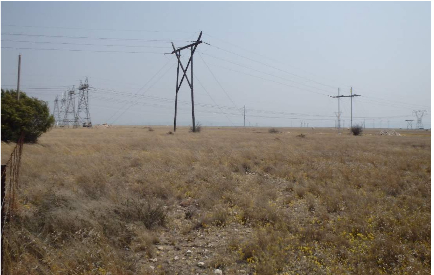
Figure 4.15: Contextual Images of Development Area indicating electrical infrastructure
