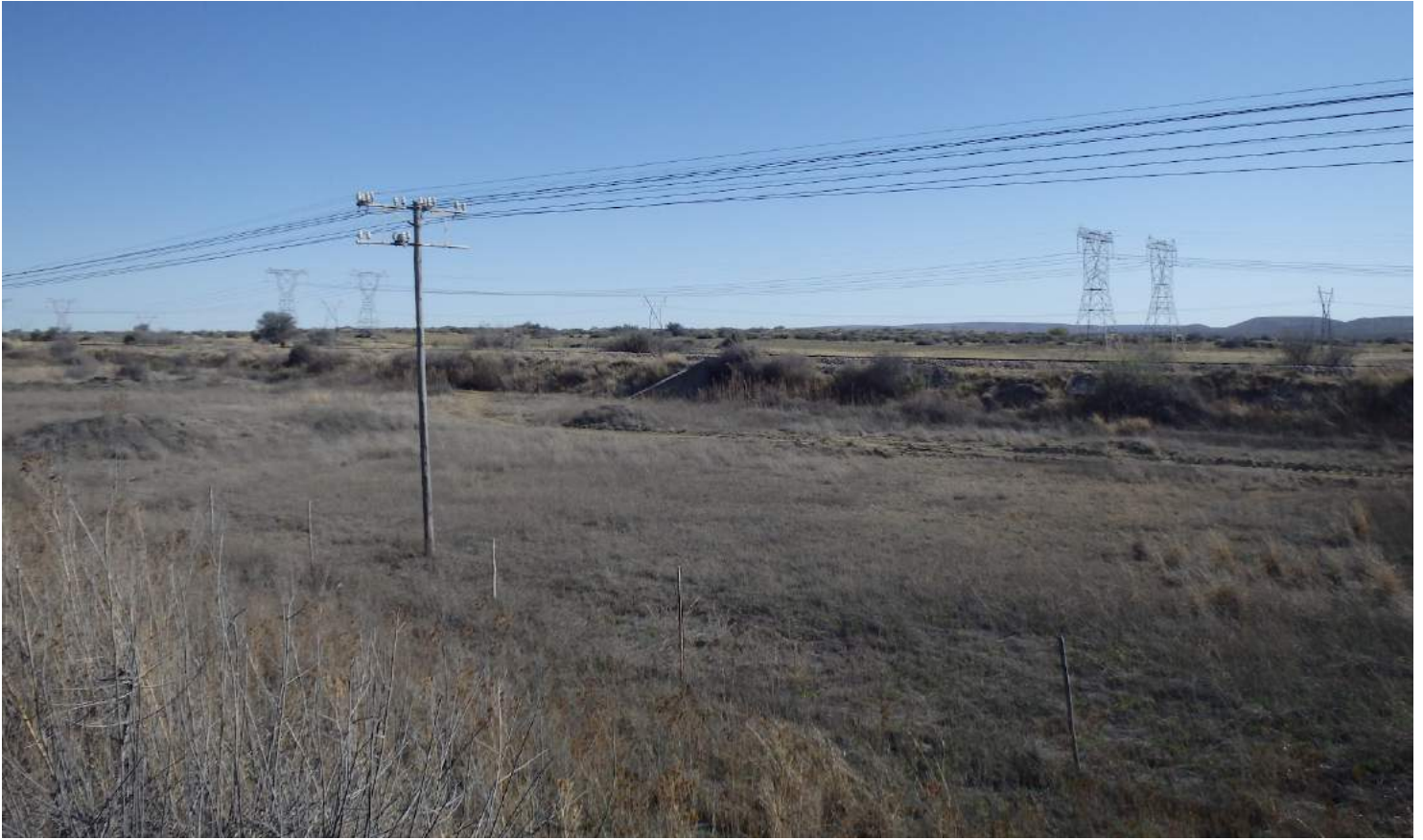
Figure 4.10: Contextual Image of the extensive OHL infrastructure.
