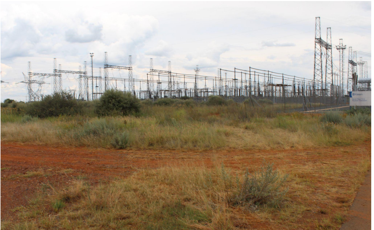
Figure 4.13 Contextual Images - Substation
