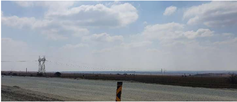
Figure 5-4: Existing 132 kV powerline extending across the site and over the R76. Photo taken at VP3 looking toward the project.
