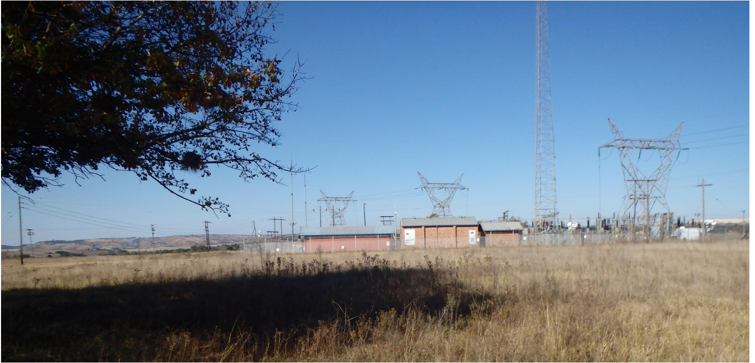
Figure 4.4: View of Tarlton substation
