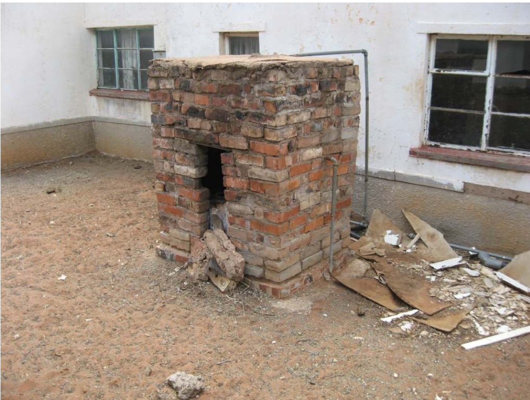
Photo 10: View of the warm water system (donkie) for the house.
