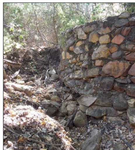
Figure 31: The undercut part of the wall.
