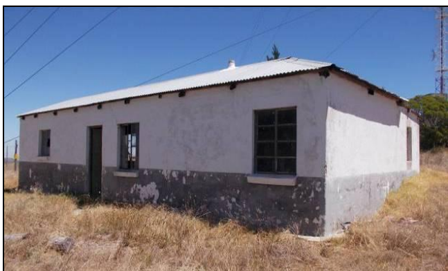
Figure 38: Mid-20 th century cottage at point 008a. It has a corrugated iron roof.
