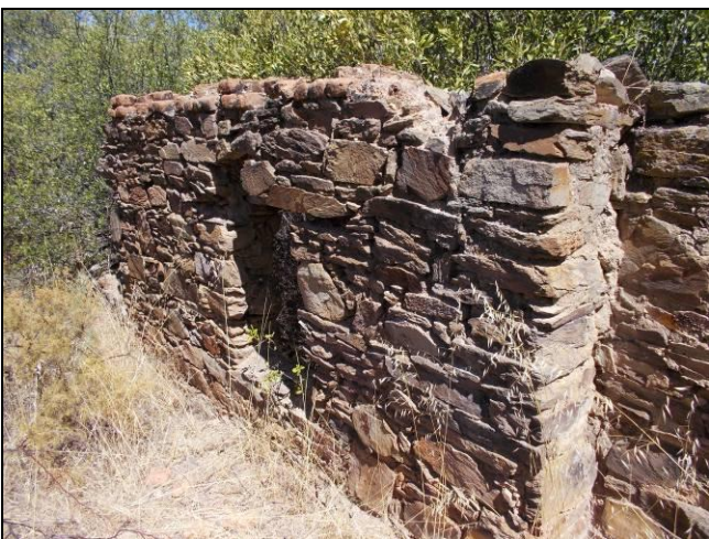
Figure 25: The west end of the northern wall of the house ruin at point 009.
