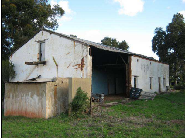
Figure 15: View of the back and north end of the 19 th century house showing the demolished section.
