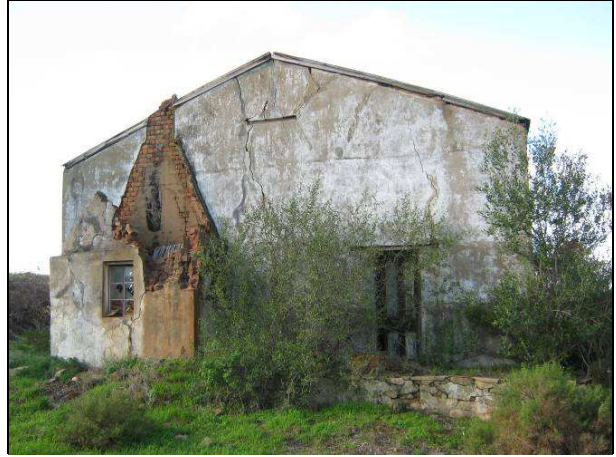
Figure 16: View of the south end of the 19 th century house showing the caved in hearth.
