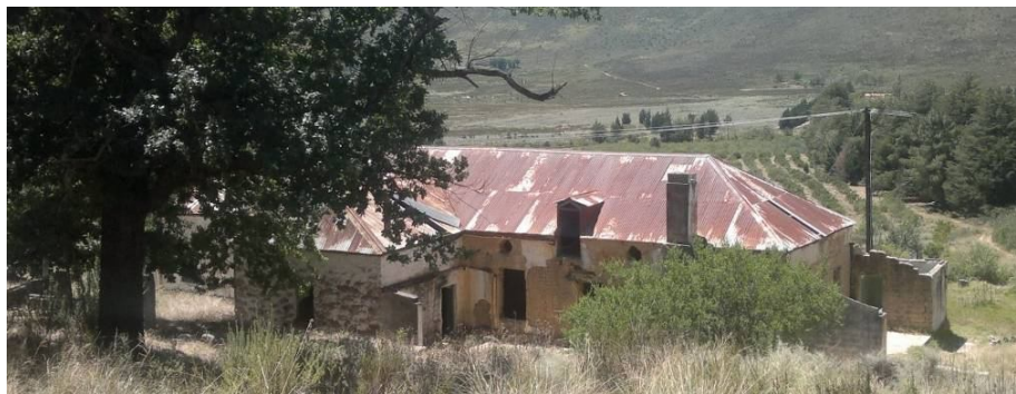
Figure 20: Back of the building with the tail addition of un-plastered stone. The central core of the building is of sun dried brickwork with clay mortar. As can be seen most of the plaster has been lost and brickwork is in poor condition
