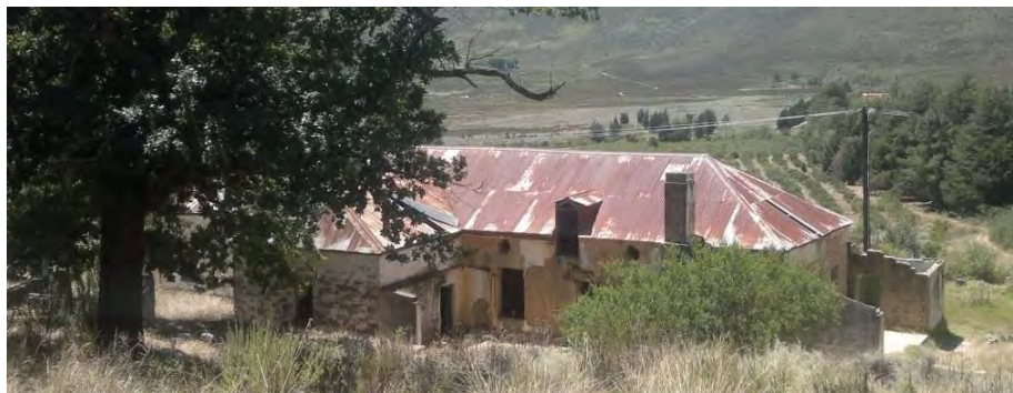
Figure 20: Back of the building with the tail addition of un-plastered stone. The central core of the building is of sun dried brickwork with clay mortar. As can be seen most of the plaster has been lost and brickwork is in poor condition
