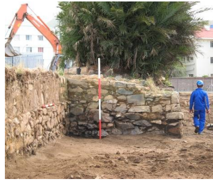
Figure 16: View of the east face of the support wall during the monitoring brief. Wall 4B is to the left of the image (the support wall abutting this wall had collapsed and was removed).
