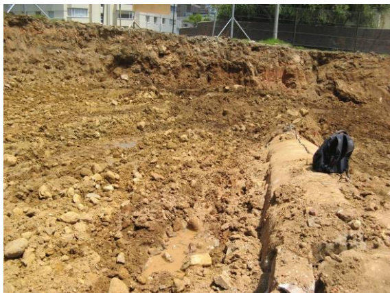
Figure 48: View of drain to the north of the substation (facing towards cnr Mount and Constitution Streets). The in situ yellow clay is clearly visible. The ground water is very high, possibly a result of the spring water no longer draining naturally nor through the constructed drain.
