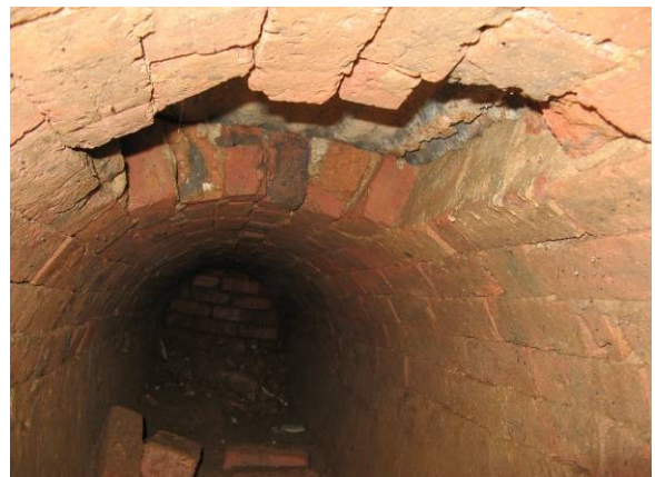
Figure 54: Repair in the same section of the drain in the form of a corrugated iron patch on the exterior.
