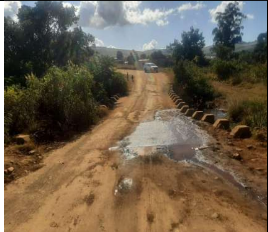
Figure 14: Picture two showing water lodging on top of the bridge and dense vegetation cover around the bridge
