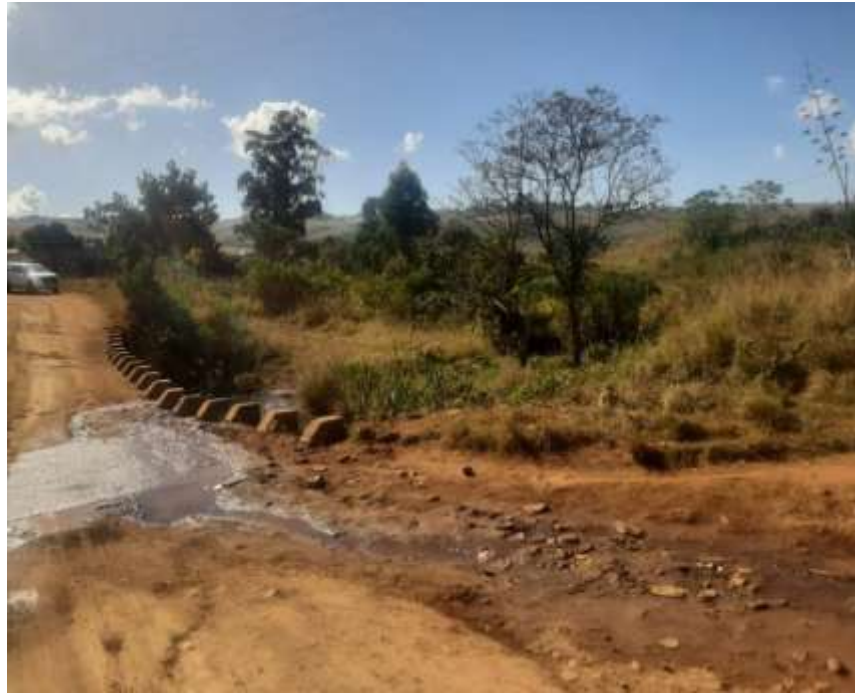
Figure 13: Picture one showing water lodging on top of the bridge and dense vegetation cover around the bridge
