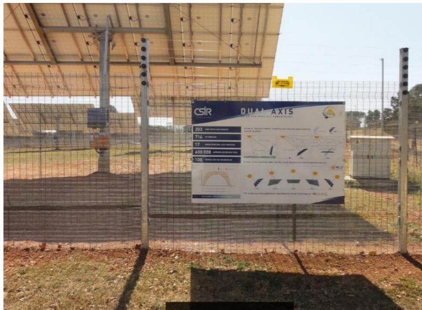
Fig 12 Explanatory board about photo-voltaic energy at the site.
