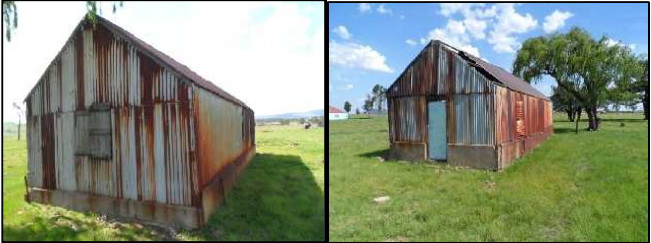
Figure 40 - Photos showing the historic corrugated iron sheet shed - front and back facades as well as sides.
