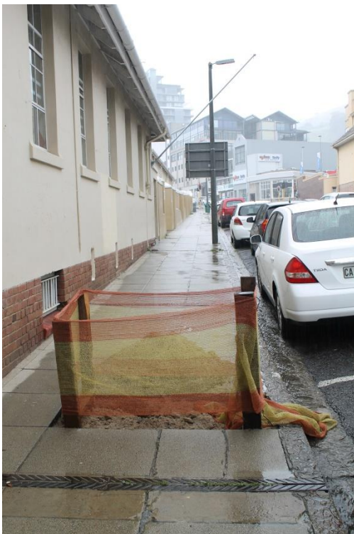
Figure 2 The first trial excavation on Chiapinni Street adjacent to the basement of the Pavement Testing Laboratory (old DRC cemetery).
