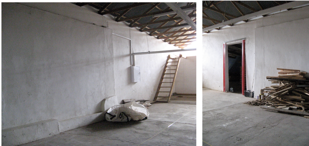
Figure 5: Views of the 'eastern end' of the 18 th century portion of the barn.
