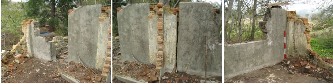
Figure 17: Brick columns forming the southern wall of the structure. The infill between the columns is of modern pink/red brick and cement mortar. The structure was probably converted to a dwelling in the early 20 th century.
