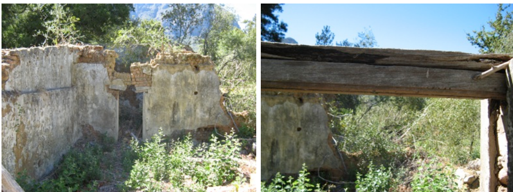
Figure 7: View of northern room of Cottage 1. Again the height of the stone walling is clearly visible. The image on the right shows the detail of the remains of one of the wooden window frames with quarter round moulding.
