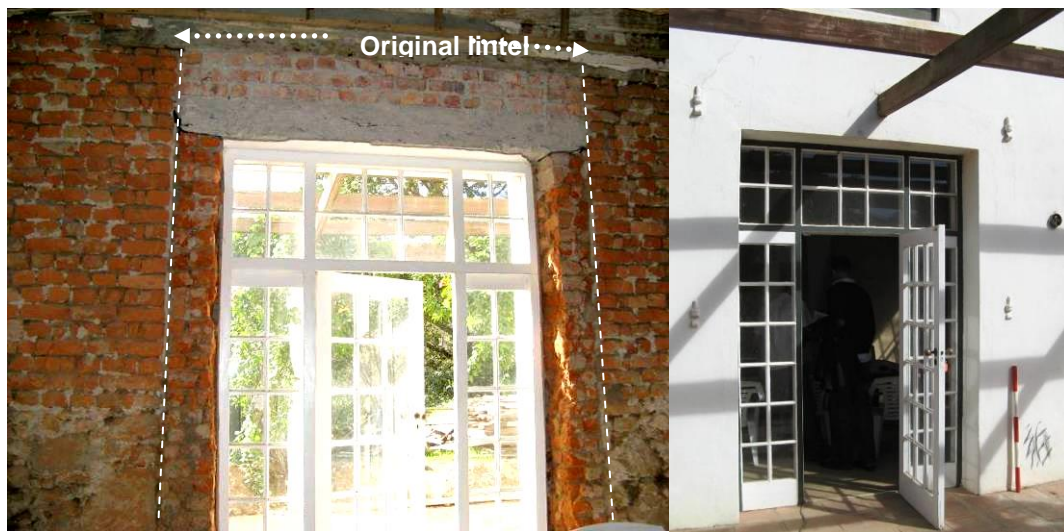
Figure 4: Door opening in eastern flank. Originally accommodating a wider double barn door (iron hinges are still visible on the outside), this is the only opening in the structure that has not been punched through existing stone walling, but built in place. The image on the right shows the same door from the exterior: note the position of the hinges.
