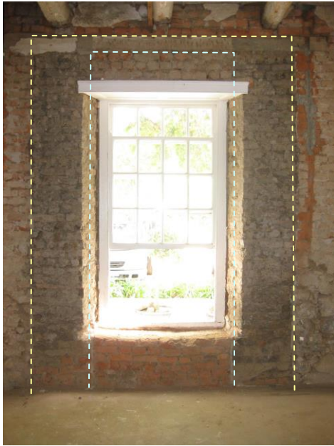
Figure 5: Door opening in northern flank beneath gable. Two alteration phases are clearly visible: 1) the narrowing of the space to accommodate a single door with fanlight and the replacement of the door with the present sash window.
