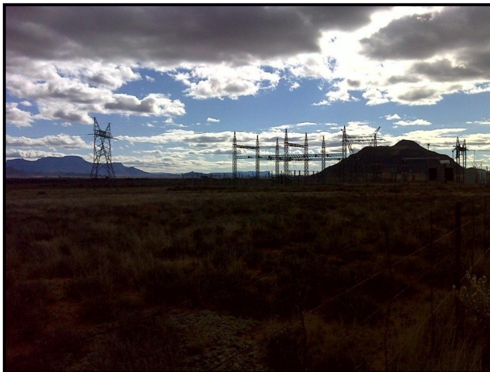
Figure 6. View of the existing Collett Substation proposed to be upgraded.
