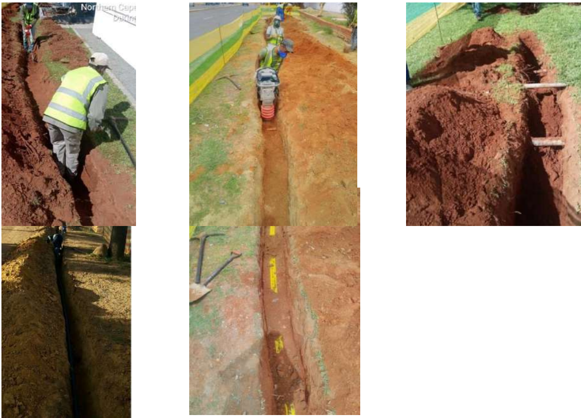
Figures 4 - 6: Some photographs of conventional trenching within the Sol Plaatje Municipal area
