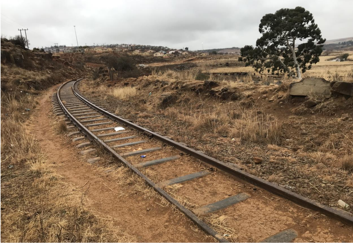
Figure 9: An overview of the railway line on the southern section of the proposed area.
