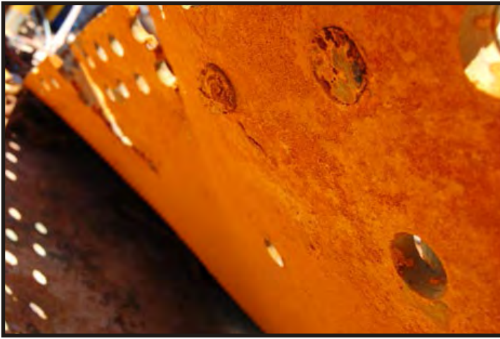
Figure 120: Flush points of pan head rivets, corrosion has bulged it slightly. (Photo V. Maitland)
