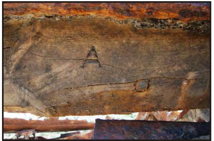
Figure 280: Ceiling marking - A (Photo V. Maitland)
