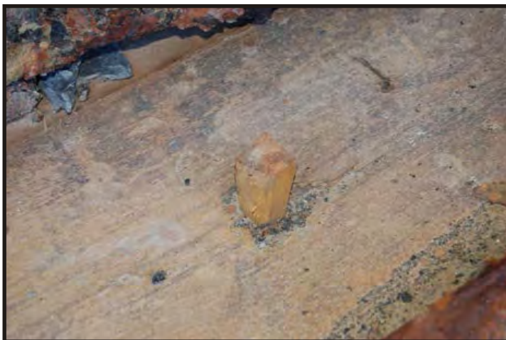
Figure 304: Wooden dowel in the hold ceiling, this one is particularly badly fitted. (Photo V. Maitland)
