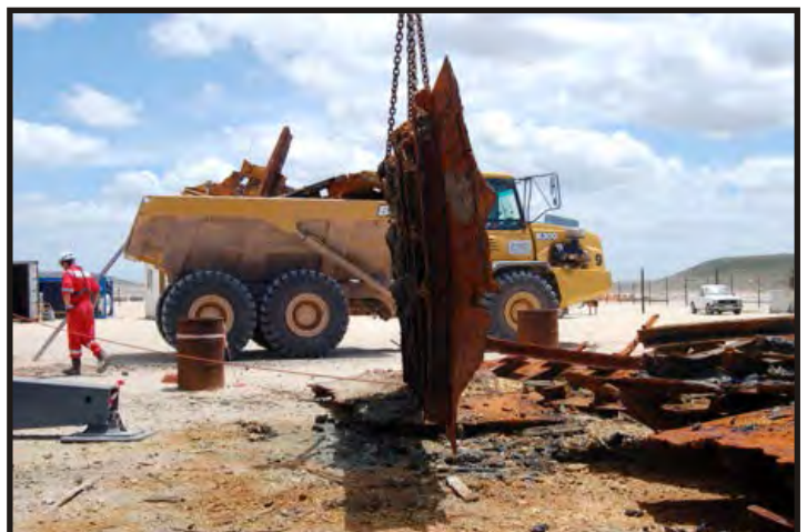
Figure 110: Side view of side plating. The in-and-out system of plating and the butt strap can be seen. (Photo: V. Maitland)
