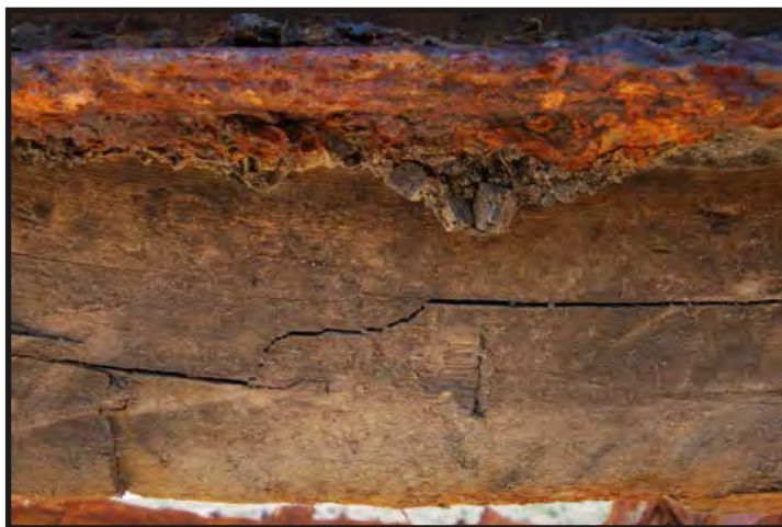
Figure 276: Ceiling marking - B I (Photo V. Maitland)
