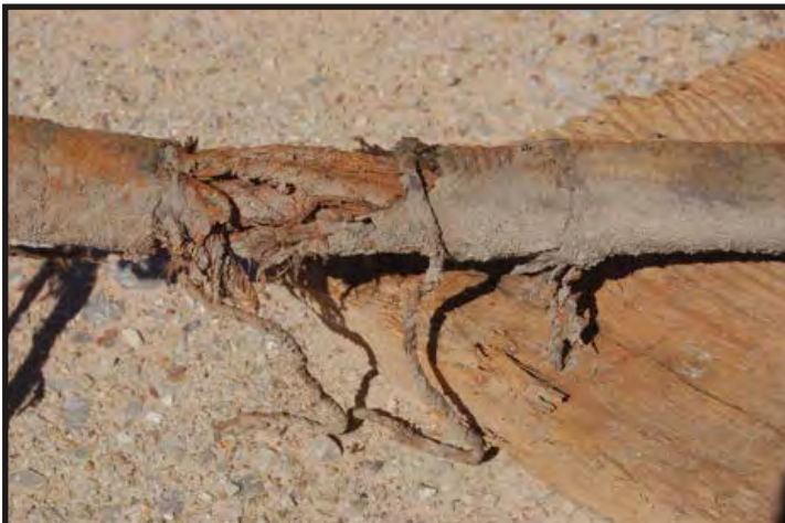
Figure 363: Section of wire rope showing the disintegrated manilla covering and exposing the wires beneath. (Photo V. Maitland)
