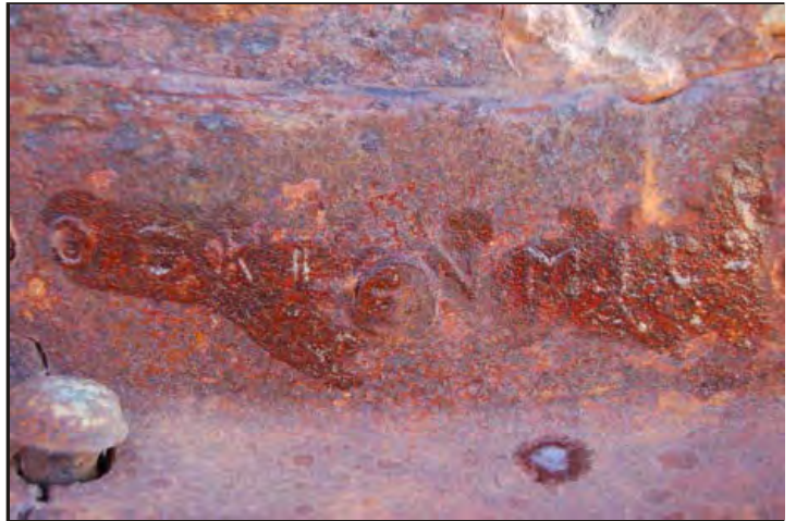
Figure 134: Manufacturer's stamp on the web framing. All that can be seen is OCKTON M IC o . The Lloyds' Survey states the iron comes from the West Stockton Iron Co, Stockton. (Photo V. Maitland)
