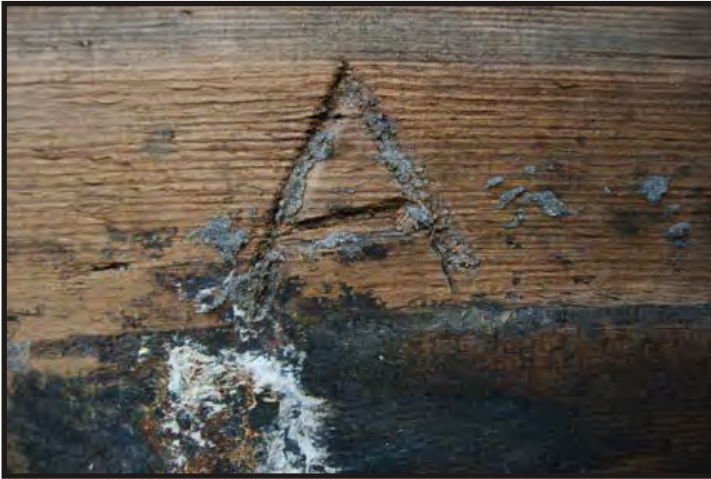
Figure 291: Ceiling marking - A (Photo V. Maitland)
