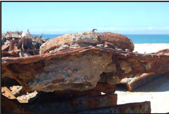
Figure 189: Side view of the lower end of the hawsepipe as it passed through the side plating. (Photo V. Maitland)
