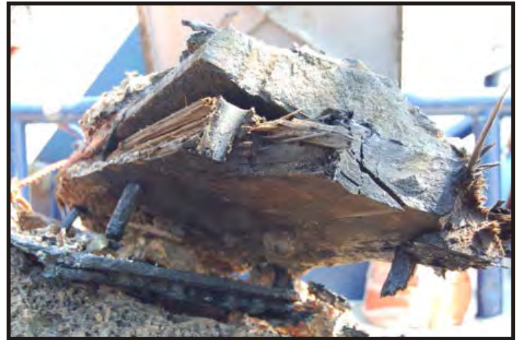
Figure 214: Close-up of beams and deck. Bolts for attaching the deck to the beam are visible. (Photo V. Maitland)
