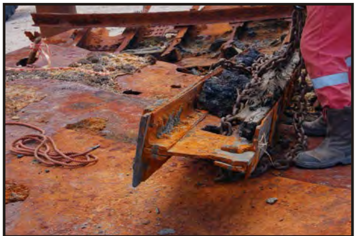
Figure 136: Detached section of the centre keelson. The structure of the built H-beam and rider plate are visible. (Photo V. Maitland)
