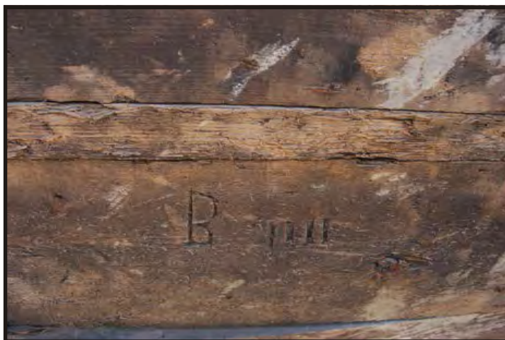
Figure 274: Ceiling marking - B IIII (Photo V. Maitland)
