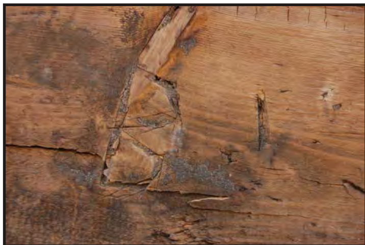
Figure 271: Ceiling marking - B I (Photo V. Maitland)
