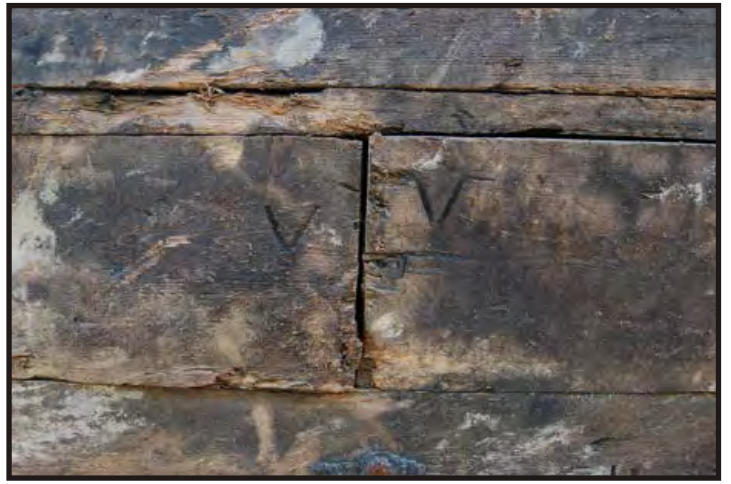
Figure 278: Ceiling marking - V V (Photo V. Maitland)
