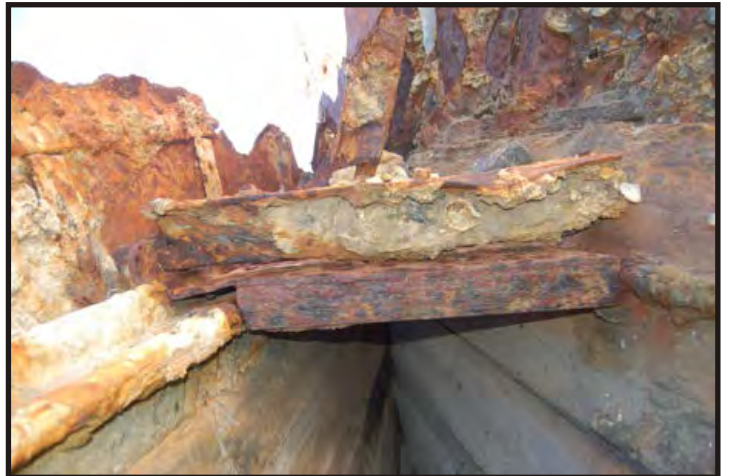
Figure 267: Close-up of the rider plate and angle iron on either side. (Photo V. Maitland)
