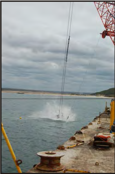
Figure 78 - 80: Crocodile grab. A crocodile grab on the Aegir barge was used to grab chunks of the wreck. (Photos V. Maitland)
