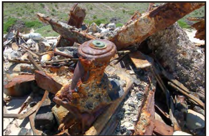
Figure 317: A different type of bollard, broken in half. While this bollard is also made of cast iron, it has a square brass bolt and 'washers' on top. (Photo V. Maitland)
