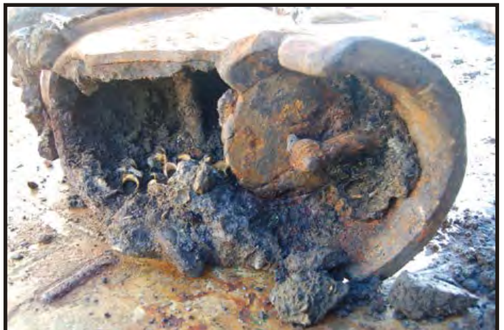
Figure 374: Top of chambered pump. (Photo V. Maitland)
