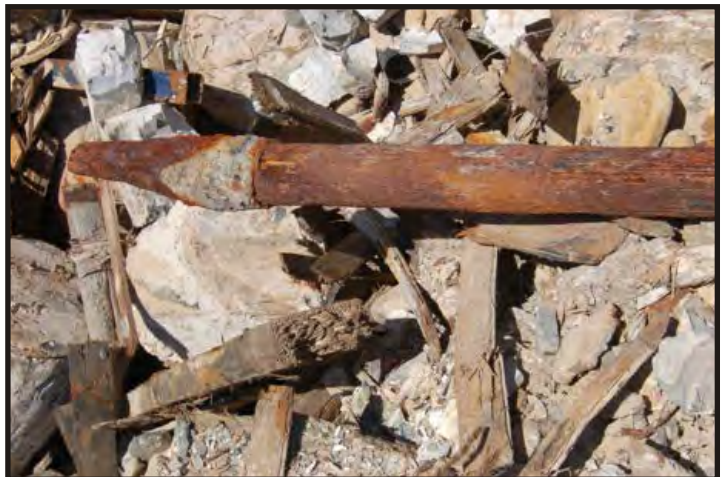
Figure 181: End of a pillar, that seems to have a sleeve attached. (Photo V. Maitland)
