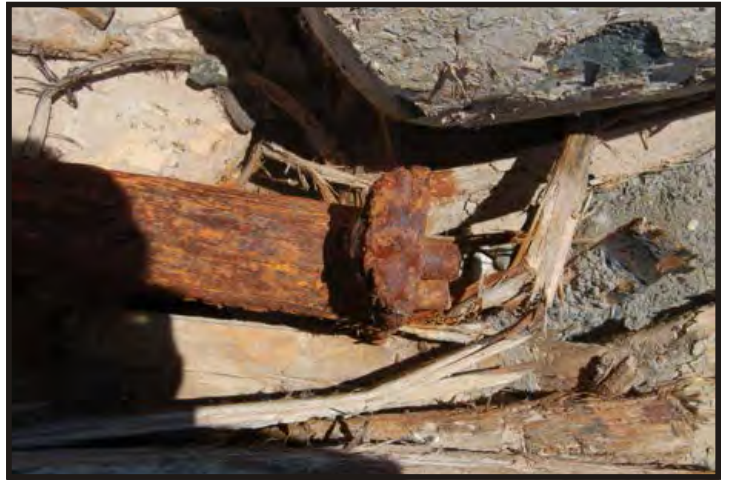
Figure 183: Heel of pillar, it is a T-section riveted to the beam or centre keelson. (Photo V. Maitland)
