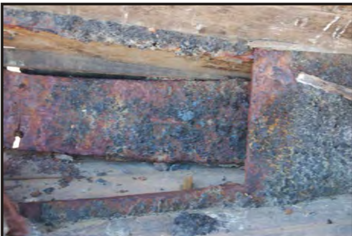
Figure 268: Top view of rider plate, which is a continuation of the side stringer and keelson. (Photo V. Maitland)
