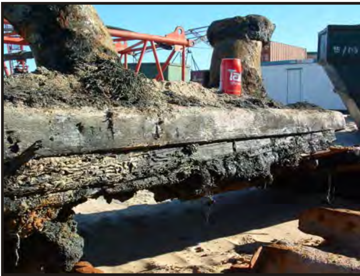
Figure 314: Close-up of the bollard, bollard plank, deck plank and rider plate. (Photo V. Maitland)
