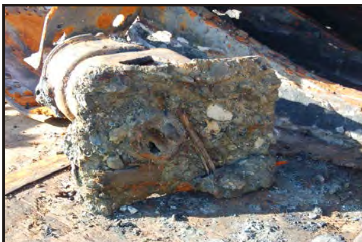
Figure 375: Bottom of pump. The pipe and remains of the deck are visible. (Photo V. Maitland)
