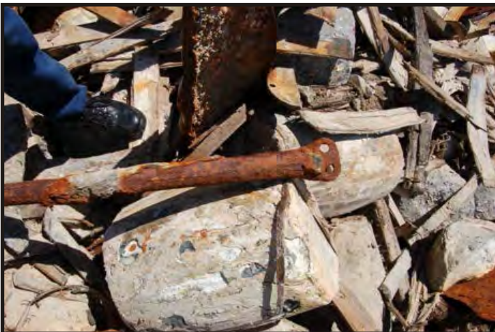
Figure 180: Head of a pillar, where it was riveted to the deck beam. (Photo V. Maitland)
