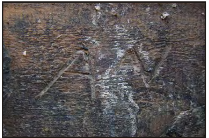
Figure 298: Ceiling marking - A V (Photo V. Maitland)
