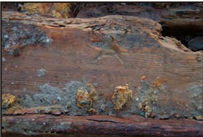
Figure 293: Ceiling marking - A (Photo V. Maitland)
