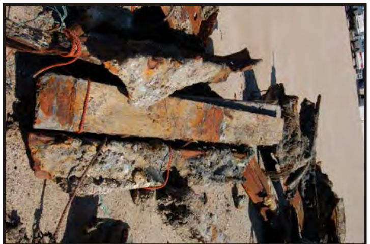
Figure 216: Bottom of a deck plank. Corrosion from the beams is visible. (Photo V. Maitland)
