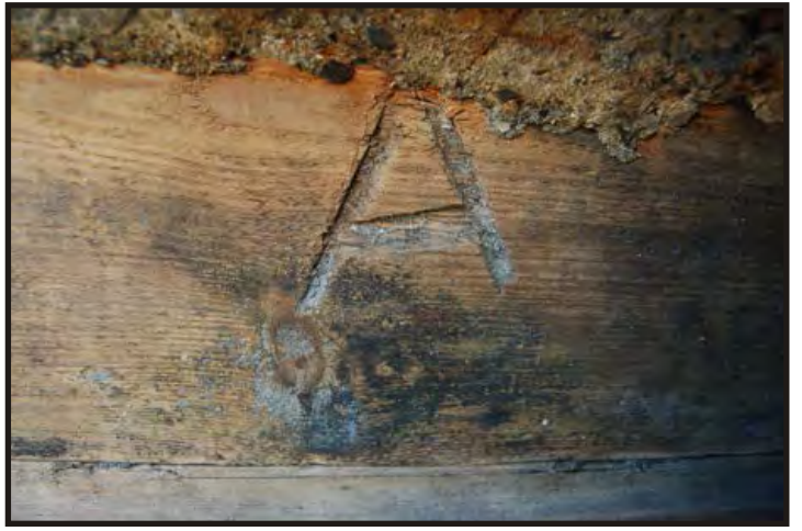
Figure 290: Ceiling marking - A (Photo V. Maitland)
