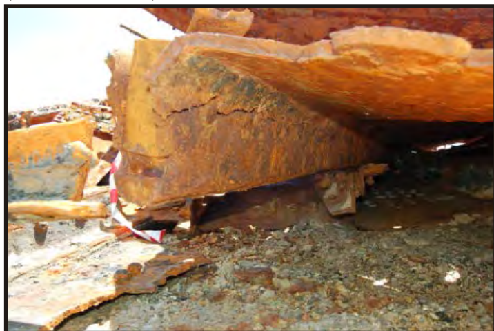
Figure 101: Bar keel from underneath, showing the corroded garboard strake. (Photo V. Maitland)
