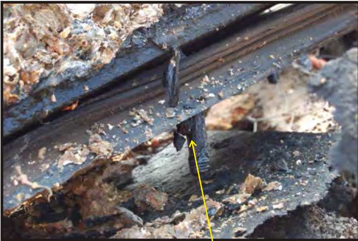
Figure 213: Close-up of beams and deck. Bolts for attaching the deck to the beam are visible. (Photo V. Maitland)
