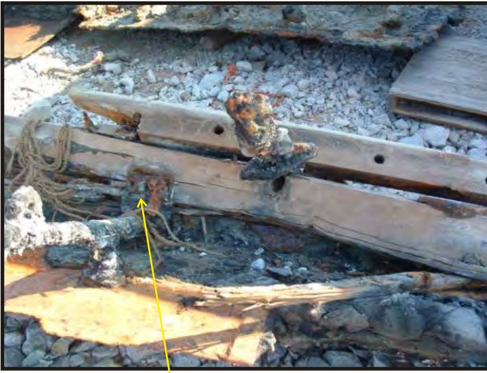
Figure 233: Bottom of channel. Note the connection of the stanchion to the bottom of the channel. (Photo V. Maitland)
