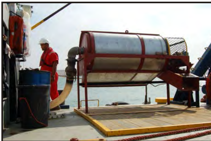
Figure 50: The 'classifier' is attached to the barge, was supposed to catch any small items dredged up. But it was not used. The debris passed through the dredge pump and the impeller broke everything up, nullifying the classifier. (Photo V. Maitland)
