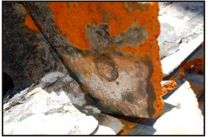
Figure 121: The point of a pan head rivet; this point is a lot less corroded and is a full point. (Photo V. Maitland)
