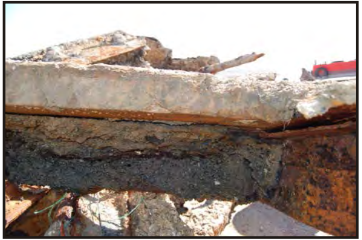
Figure 212: Side view of deck beams with the wooden deck attached. (Photo V. Maitland)
