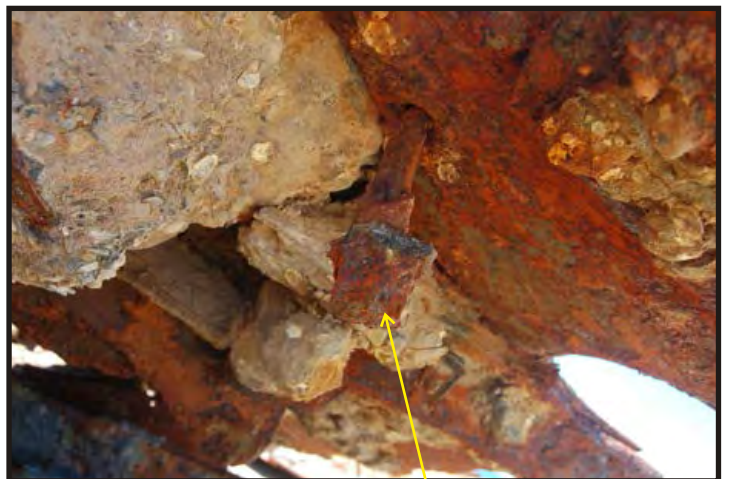
Figure 192: Close-up of lower end of hawsepipe on the inner surface of side plating. The rivet is visible. (Photo V. Maitland)
