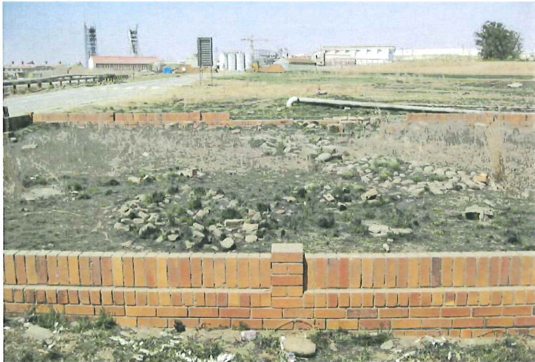
Figure 31. 'Modern' brick wall surrounding 11 graves in graveyard 14. The ironwork built into the wall was removed by thieves.
