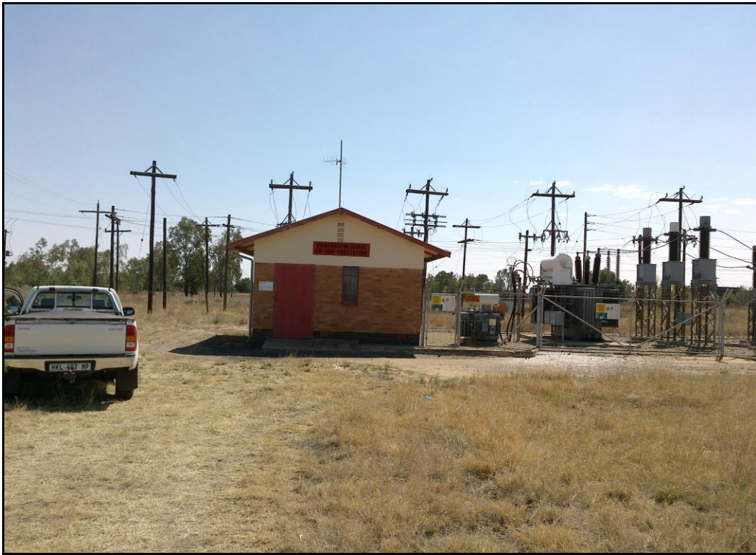
Figure 9: View of Vierfontein Rural Substation (GPS S27 05'34.7" E26 46'31.0").
