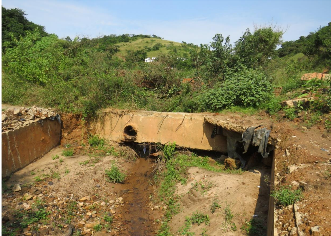
Figure 7: Damaged culvert with homestead in background
