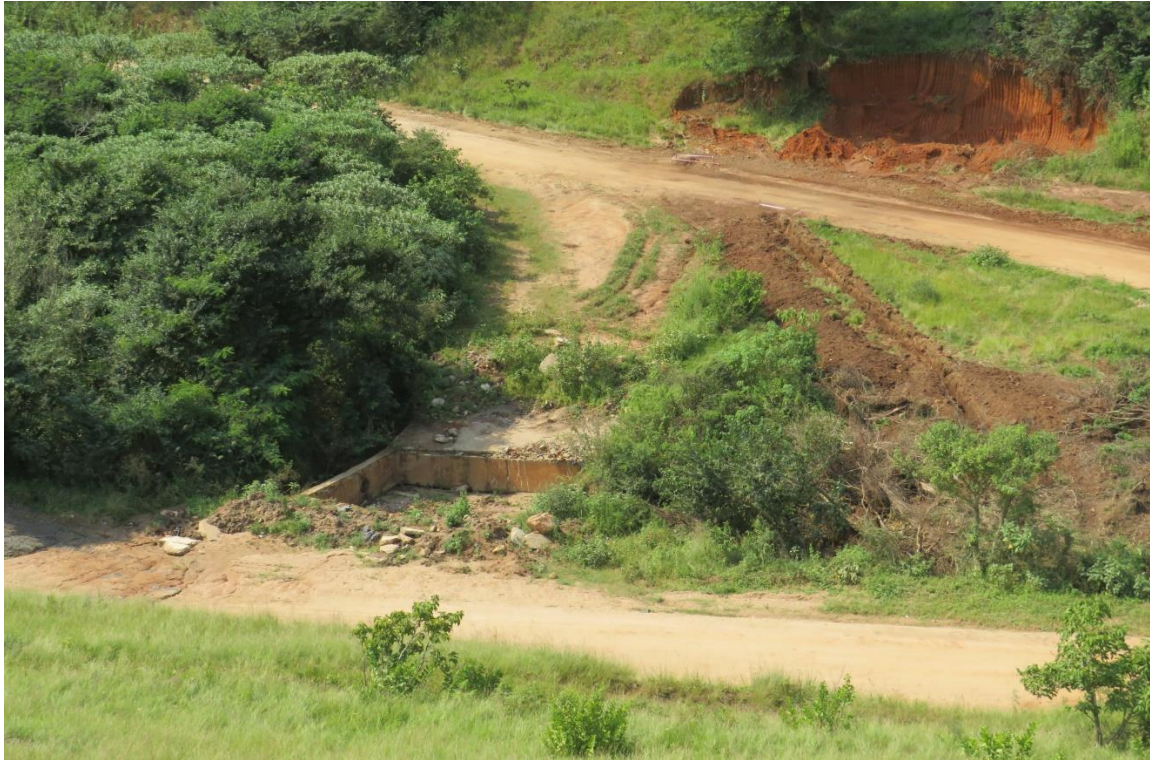
Figure 9: Damaged culvert and furrow
