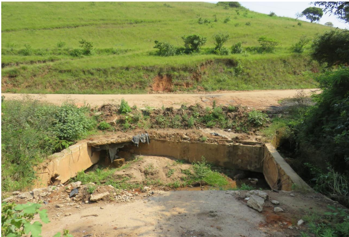
Figure 8: Damaged culvert with road in background
