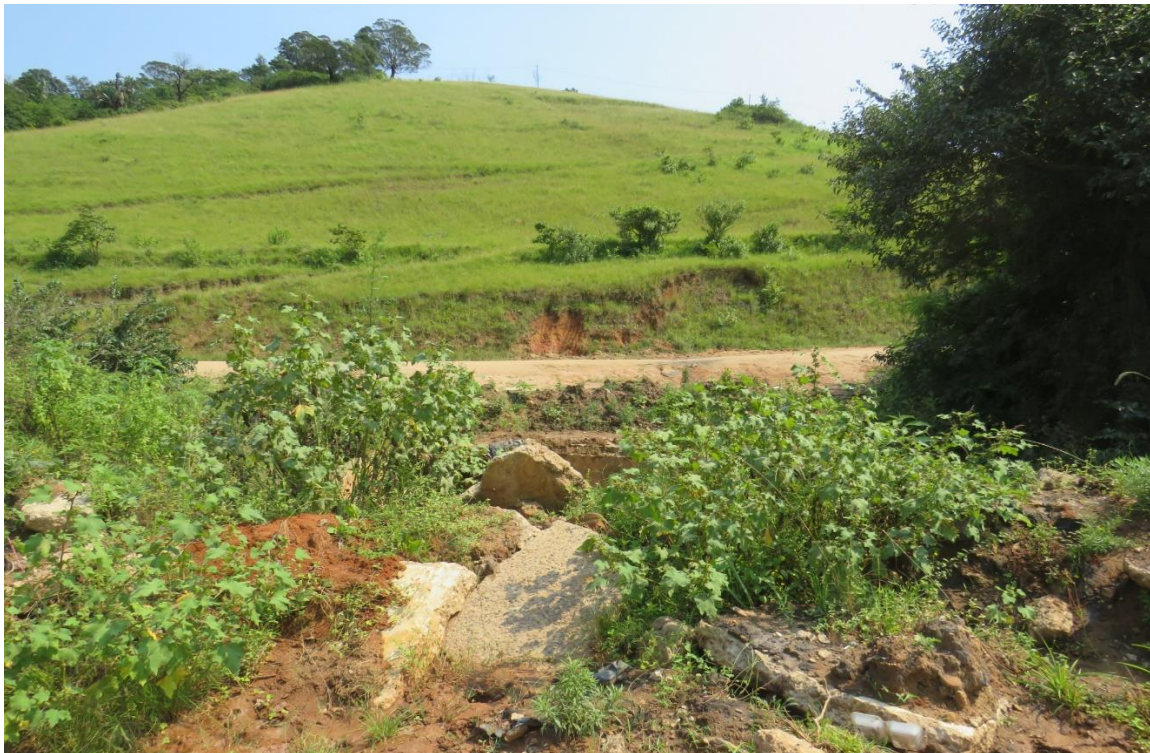
Figure 10: Remains of culvert
