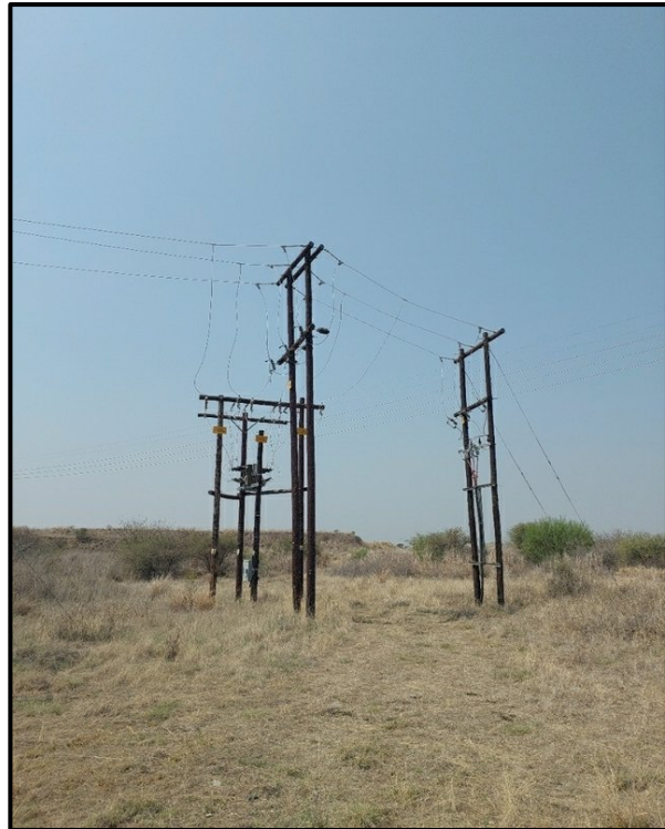
Figure 7.10. Existing smaller powerlines running across the project area.
