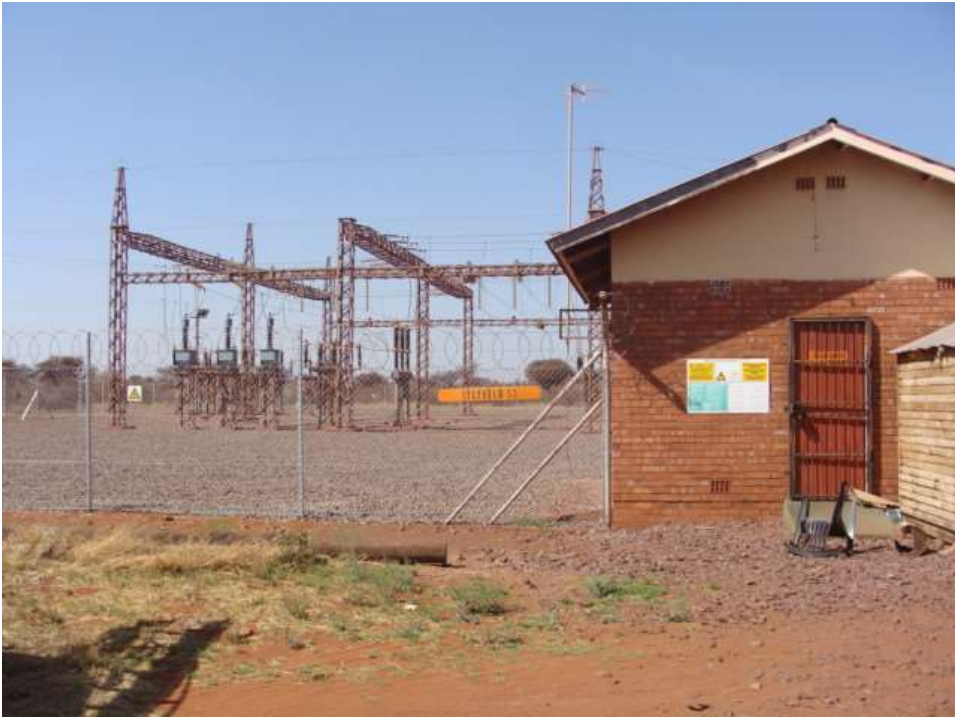
Figure 17: The Lyleveld substation towards the south of both route alternatives.
