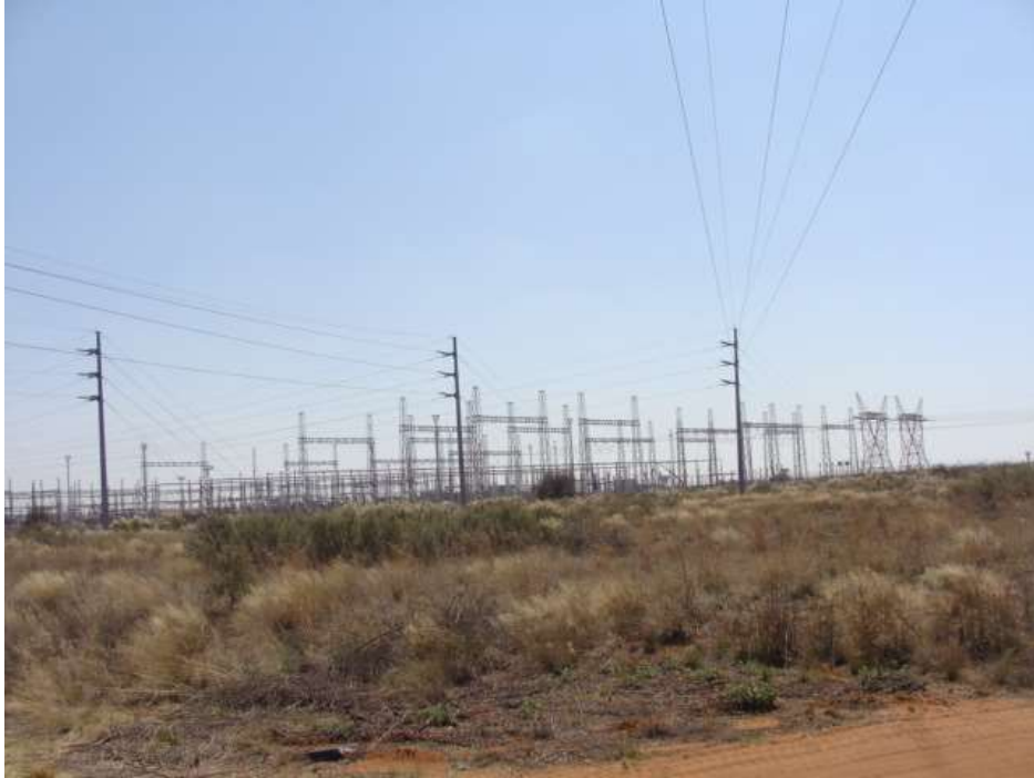
Figure 16: The Ferrum substation towards the north of both route alternatives.
