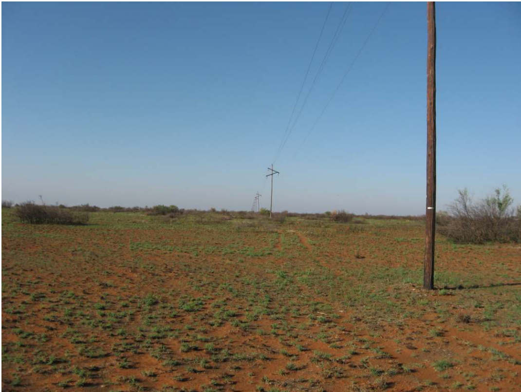
Photo 4: View of the other power line across the site.
