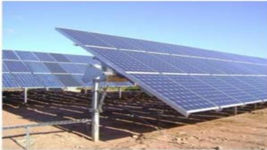
Figure 7: Example of PV Panels installed
