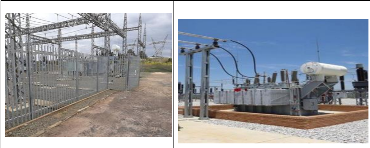
Figure 9: An Example of a Substation Picture
