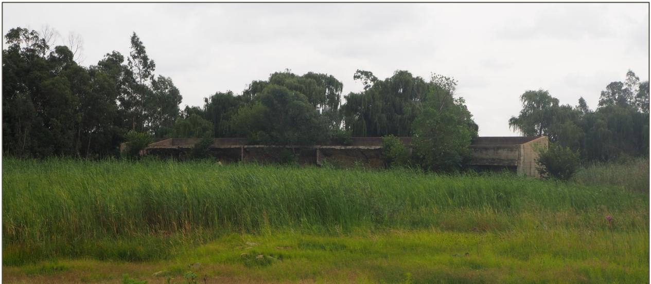
Figure 26. Dilapidated Mining Infrastructure
