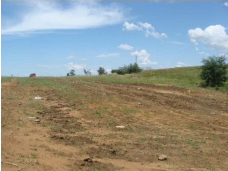
Figure 5: Further view of a section of the area where the pipeline has impacted.
