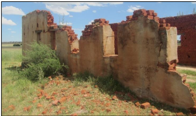
Figure 17: View of the main shed section of the ruined structure at waypoint 720. The smaller section lies to the right of this view.
