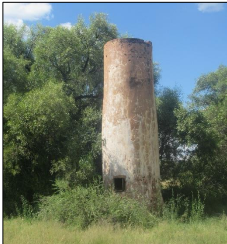
Figure 27: Ruined structure at waypoint 728.
