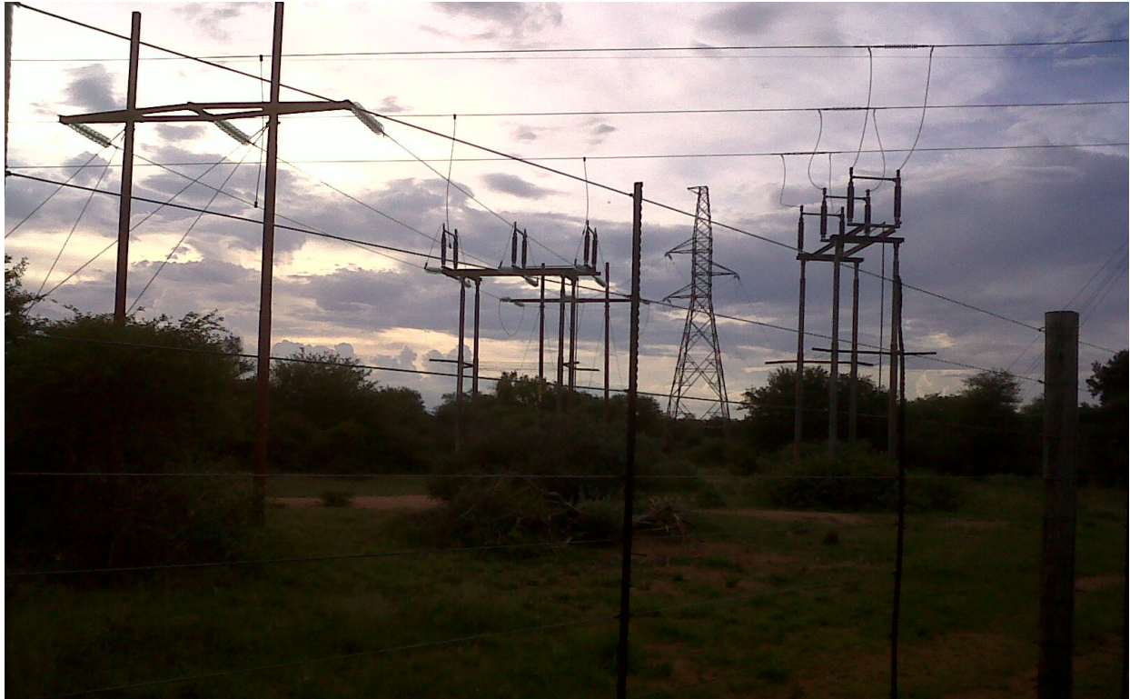
Figure 13: 132kV power line crossing the site (Thabazimbi Combined - Waterberg 1)
