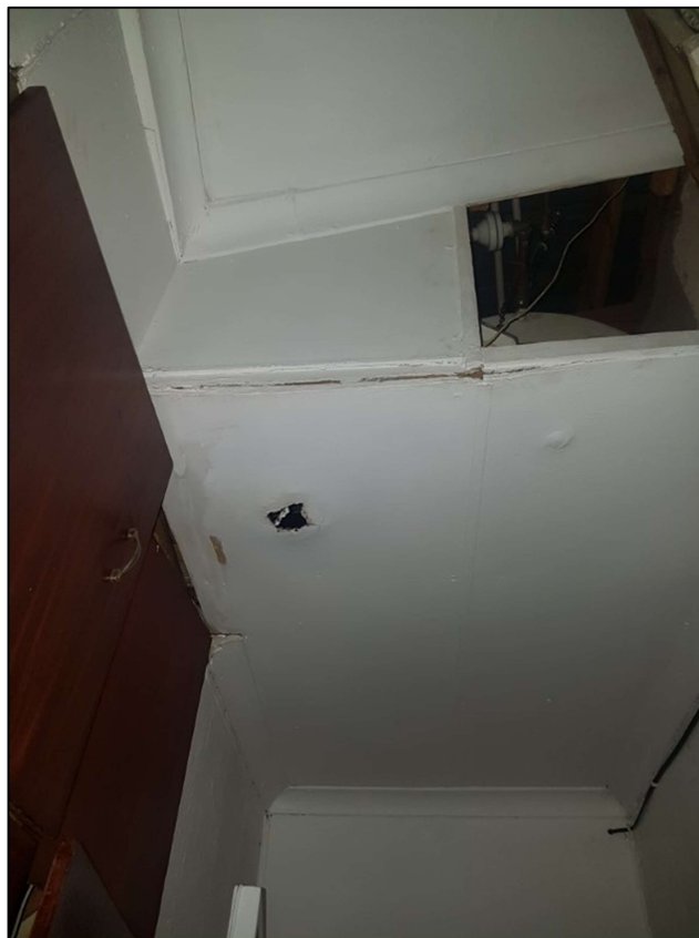
Figure 16: Damage to the ceiling.
