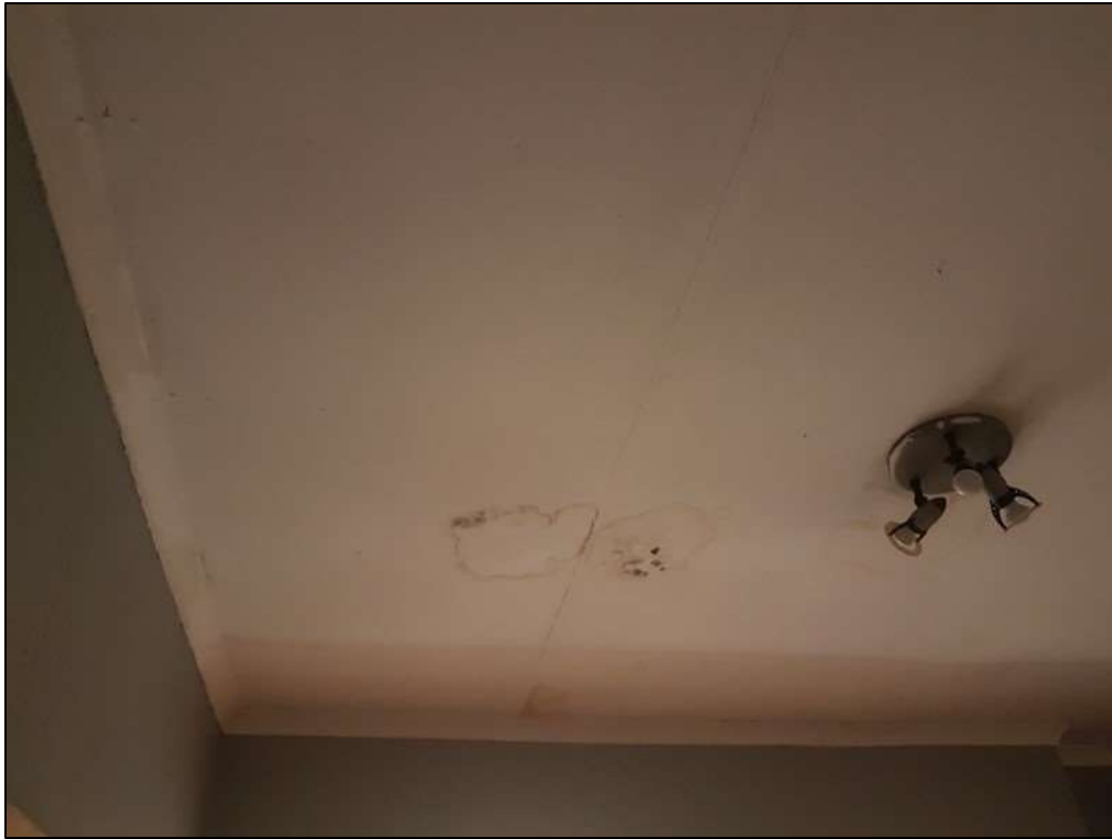
Figure 15: Water damage on the ceiling.
