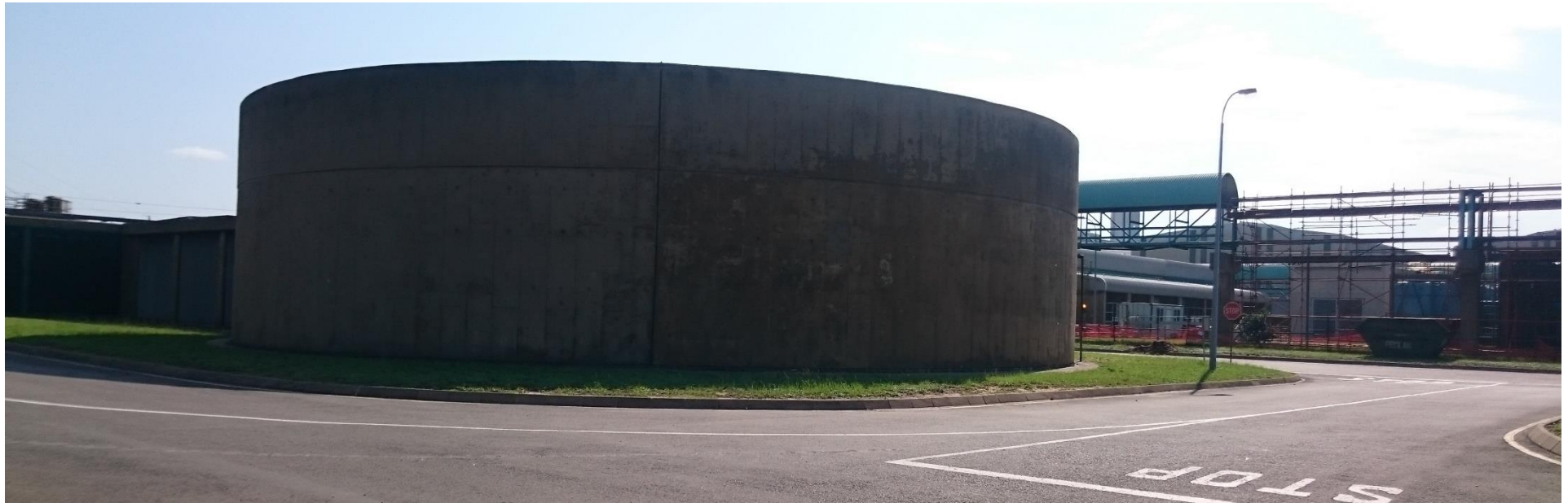
Figure 10: Hillside Aluminium process water reservoir. Process water from the proposed desalination plant will be pumped to this reservoir before being distributed within the smelter.
