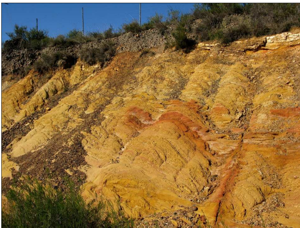
Fig. 17. Highly-weathered heterolithic zone within the Lower Bokkeveld Group with steeply dipping sandstone and mudrock interbeds, R62 road cutting (Loc. 048). Note mantle of gravelly brown soil here.
