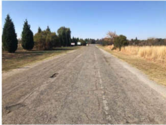
Kowie Street's road surface
